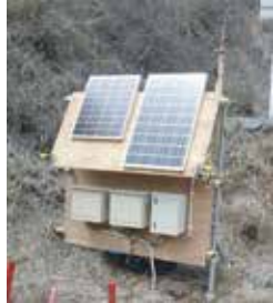
Converter Communication device (Solar battery)
